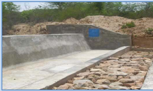
Name of the project: Pulumamidi Name of the district: Rangareddy Incomplete check dam – Non-clearance of excavated soil
